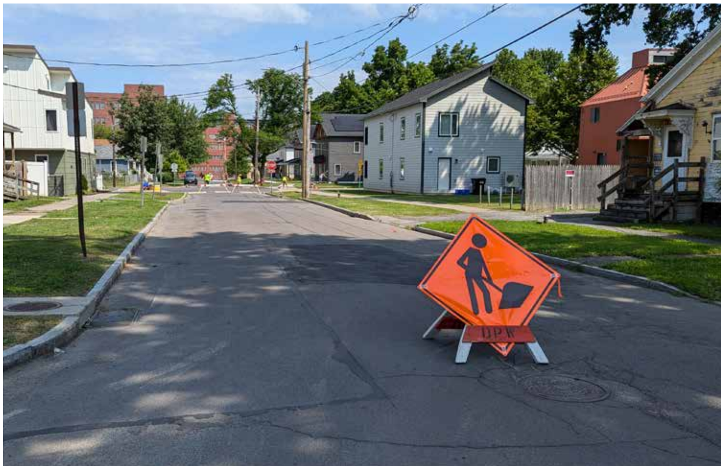
Temporary traffic control signs utilized during the installation of the Alchemical Nursery project.
