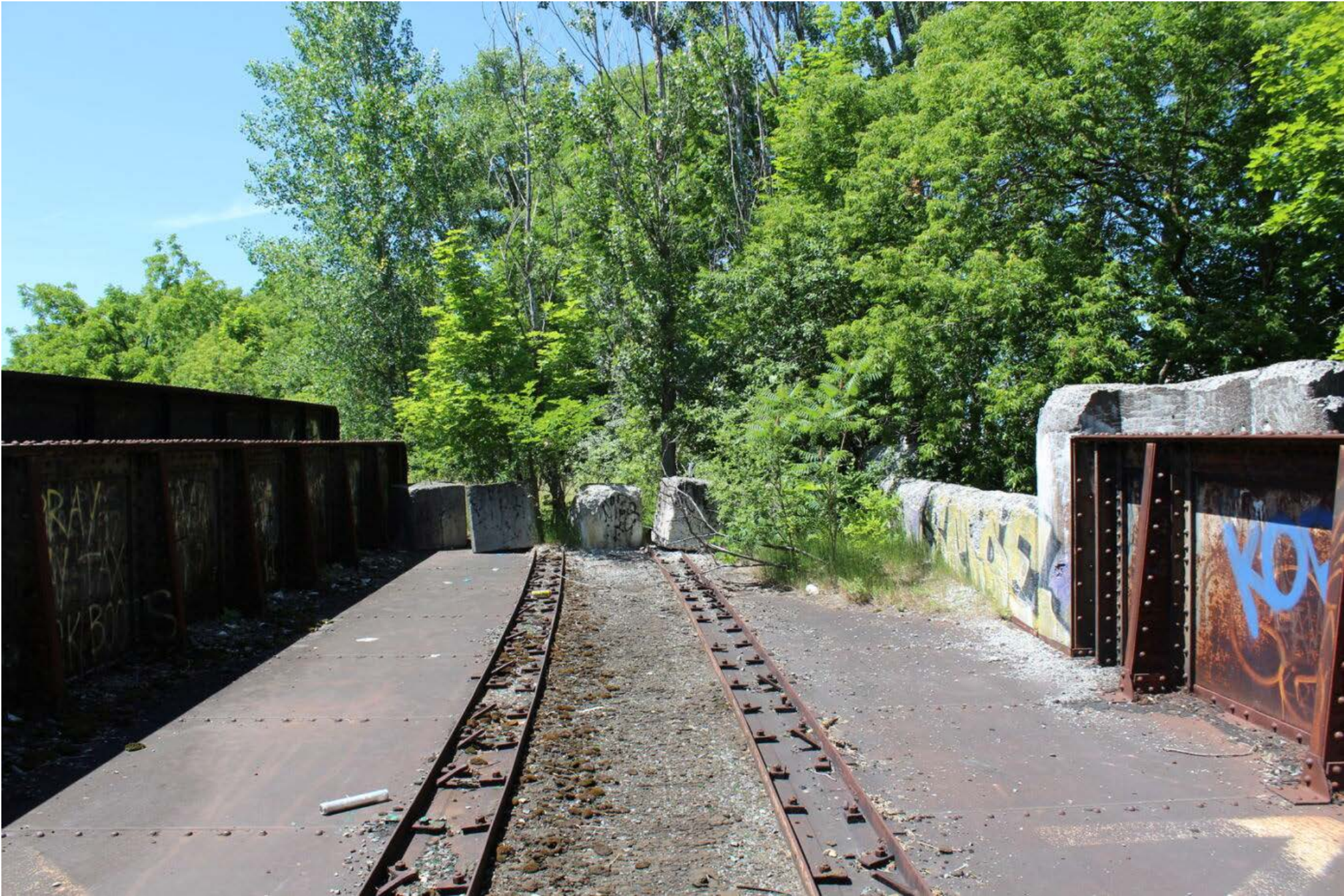
Abandoned Railroad Bridge over W Fayette St
