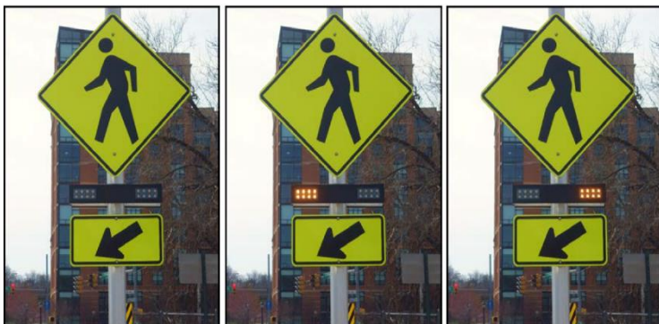
Image 19: Example of an RRFB dark (left) and illuminated during the flash period (center and right) mounted with W11-2 sign and W16-7P plaque at an uncontrolled crosswalk. Source: FHWA Interim Approval for Optional Use of Pedestrian-Actuated Rectangular Rapid-Flashing Beacons at Uncontrolled Marked Crosswalks, 2018.
