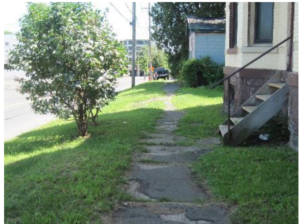
Existing sidewalk on West Fayette Street is not compliant with ADA standards or City codes.
