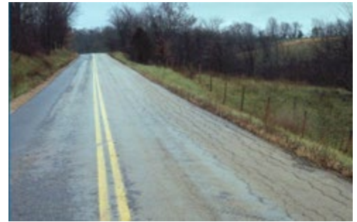
Distress, such as cracking, is frequent and severe on roads with “poor” pavement condition.
