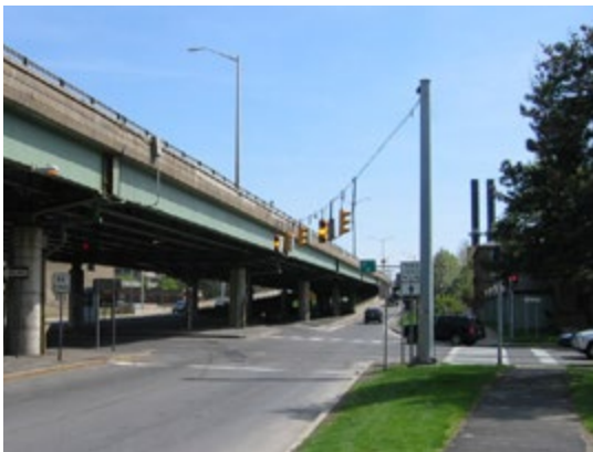
The future of the aging I-81 viaduct in downtown Syracuse continues to be the subject of extensive local planning efforts.
