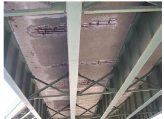
Deterioration is visible on the underside of this bridge deck.
