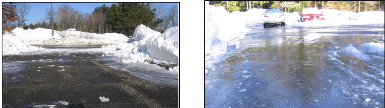
Figure D-4 - Porous asphalt (left) and dense mixed asphalt (right) parking lots shown after a spring rain on snow event Source: University of New Hampshire Stormwater Center
