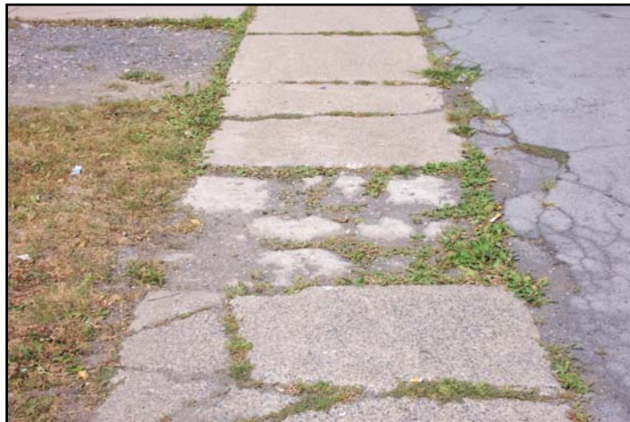
Poor sidewalk conditions can hinder pedestrian mobility.
