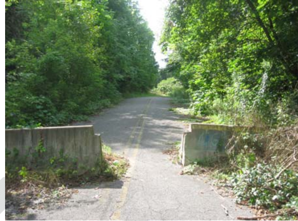
Image: Closed Roadway - Valley Drive, Town of Elbridge (Elbridge R1). Description: A section of Valley Drive along Skaneateles Creek is closed between the villages of Elbridge and Jordan.
